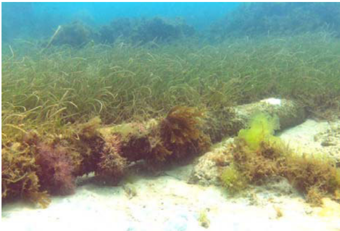
Existing cable (under water pictures)
